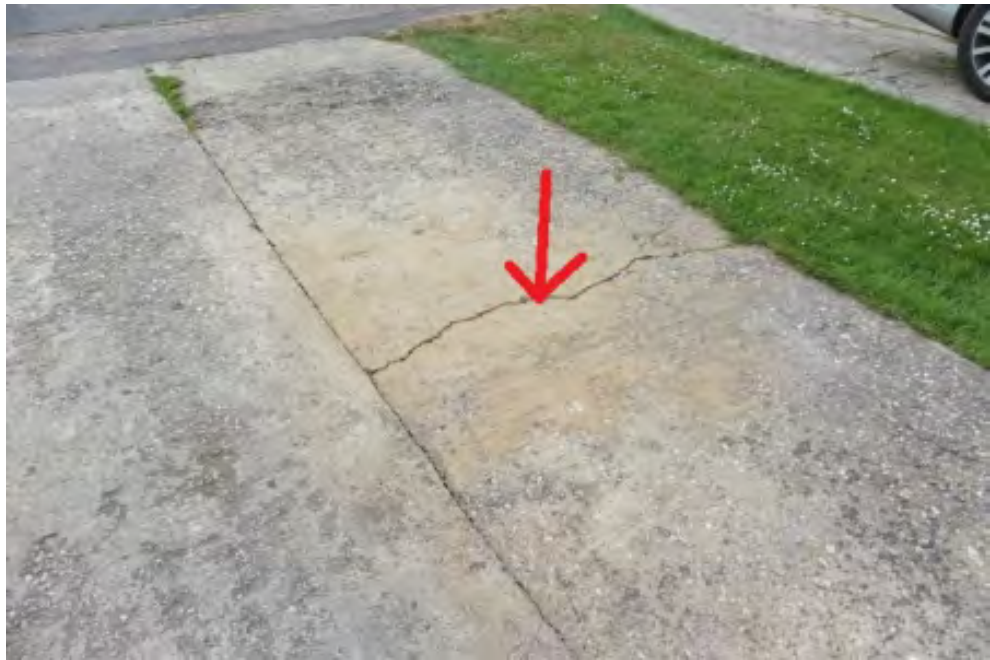
Cracking in the front drive
