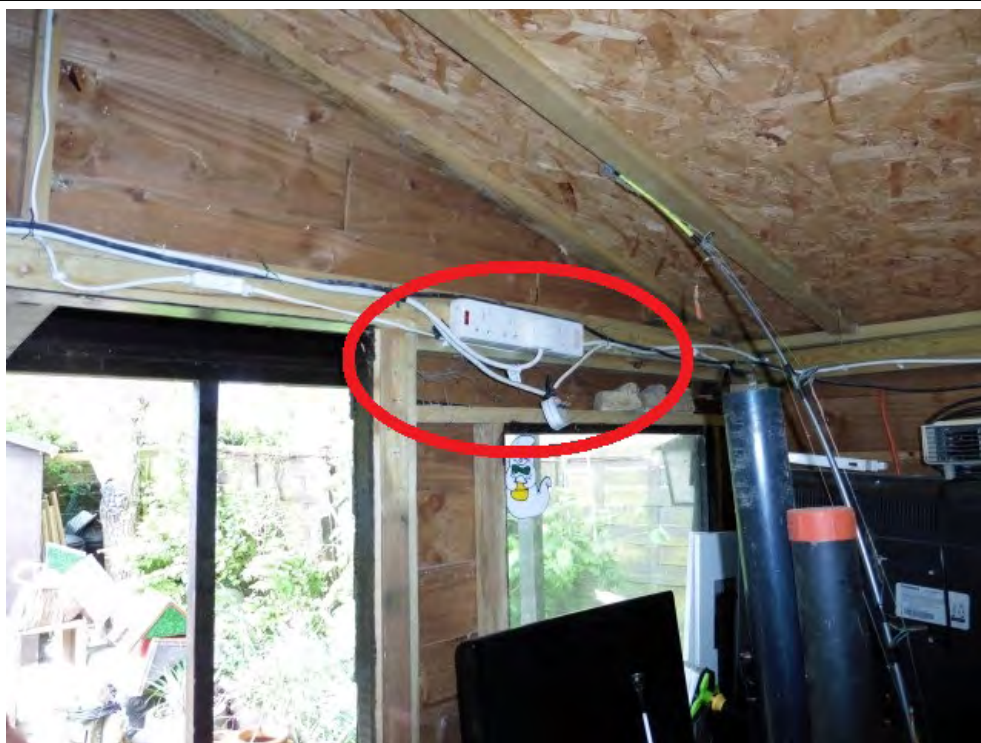
Poorly managed wiring in shed 4
