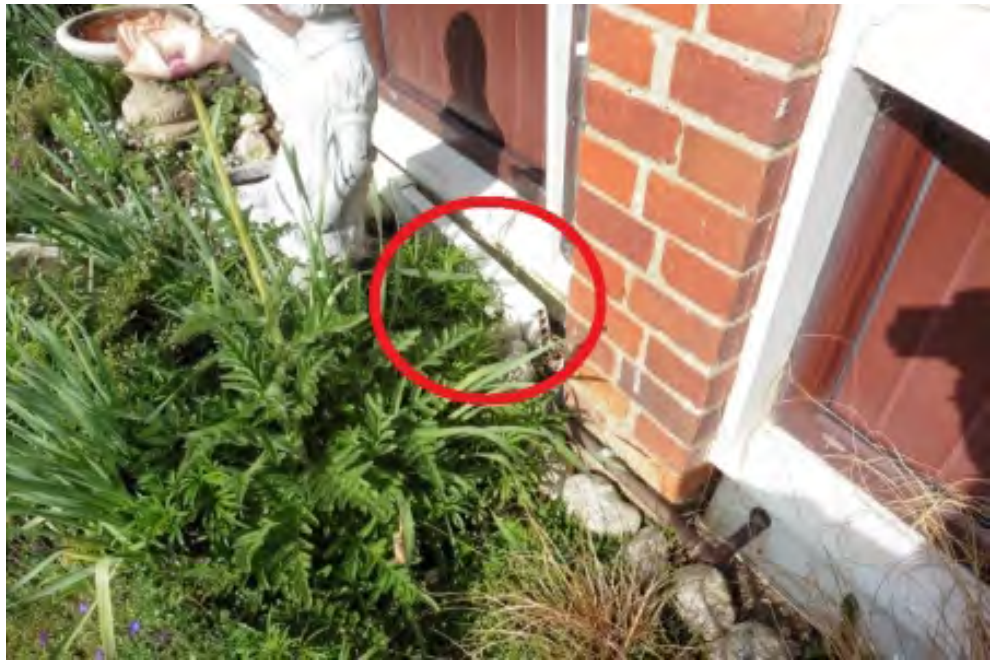
Loose plastic trim at the front
