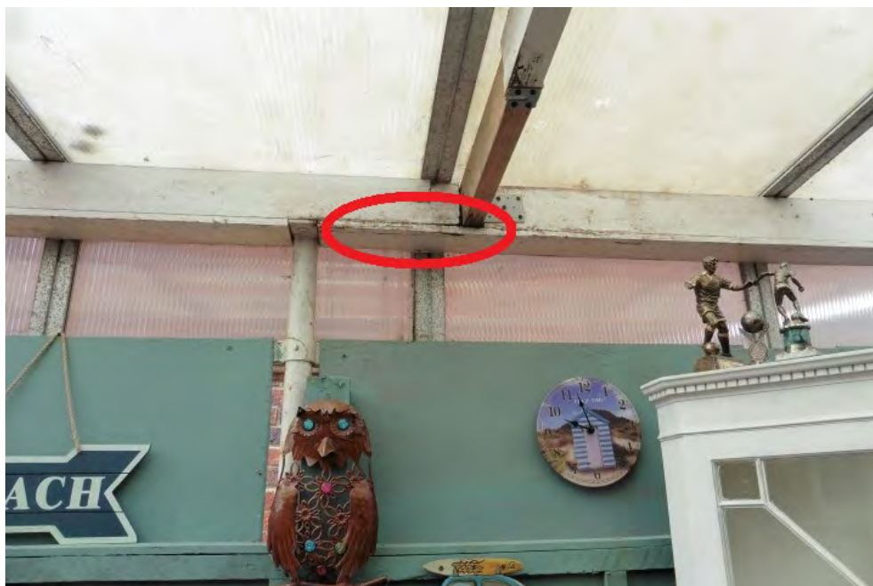
Possibly rotten timbers in the lean-to
