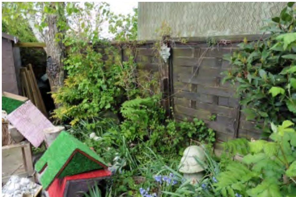
Rear boundary fencing maybe loose
